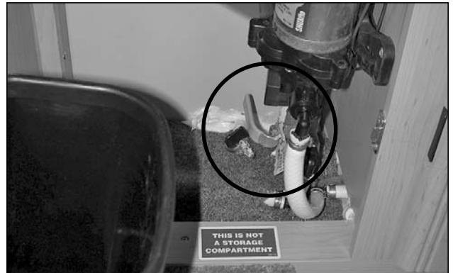
Picture G-P7: Interior tank drain valve in closed position.
